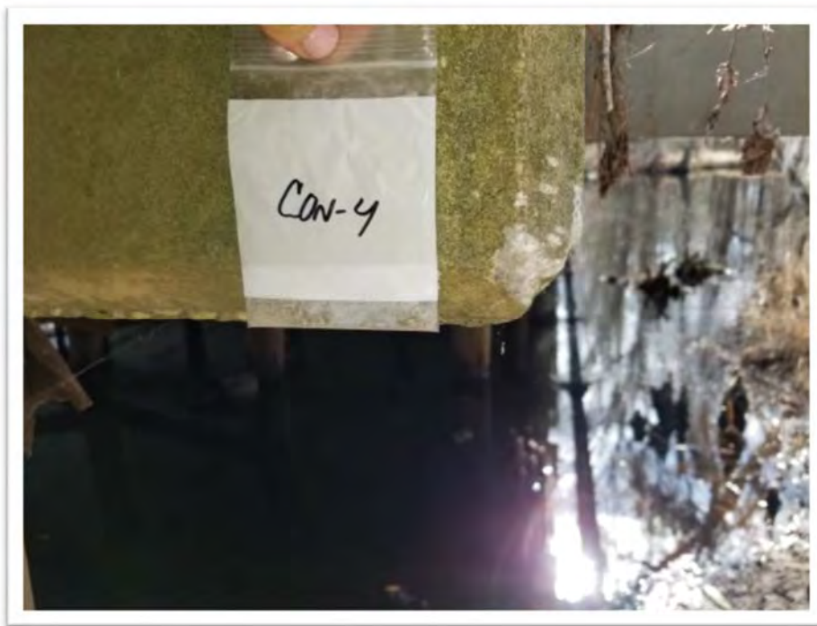
Photograph #20 Sample CON-4 – View of Concrete Sampling Point on a Beam on the Underside of Bridge 3 (None Detected)
