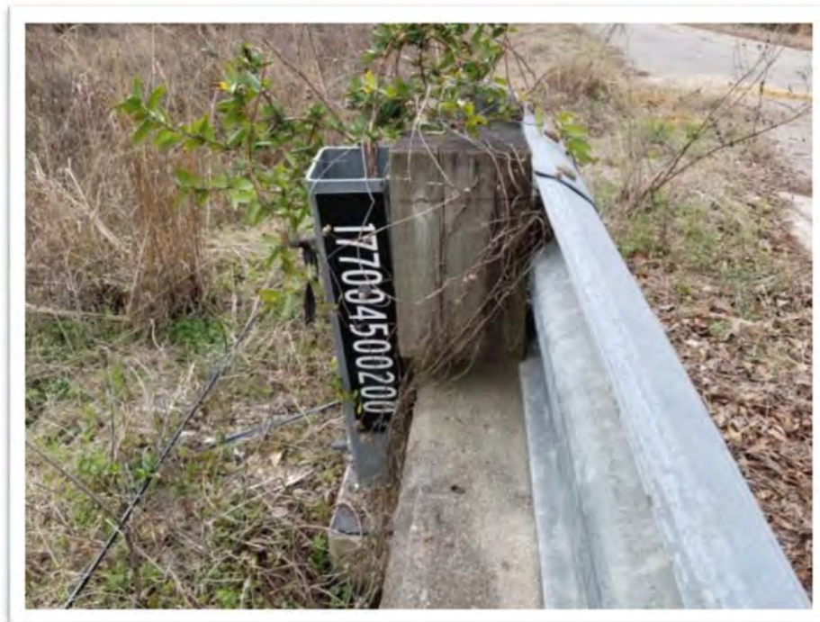
Photograph #02 View of Placard on Bridge 2 – Bridge 2 is Located Over the Middle Section of the Little Pee Dee Swamp
