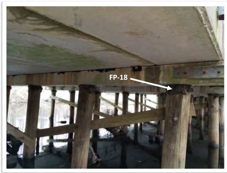
Photograph #14 Sample FP-18 – Felt Paper Sampling Point Located Between Wood Bent and Concrete Beam on Bridge 2 (None Detected)
