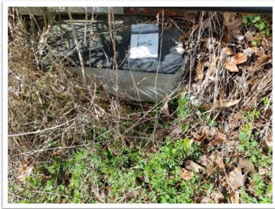
Photograph #11 Sample BM-16 – Black Bearing Pad Sampling Point Between the Deck of Bridge 2 and the Abutment at the North End of the Bridge, East Side (None Detected)
