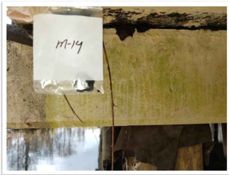
Photograph #10 Sample M-14– Black Mastic Sampling Point Between Concrete Beams and the Black Bearing Pad on the Underside of the Deck on Bridge 2 (None Detected)
