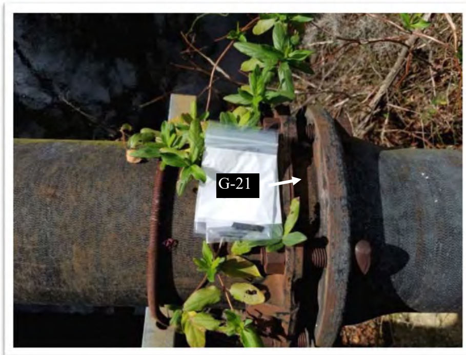
Photograph #12 Sample G-21 – Rubber Gasket Sampling Point on the Water Line Parallel to the West Side of Bridge 2 (None Detected)
