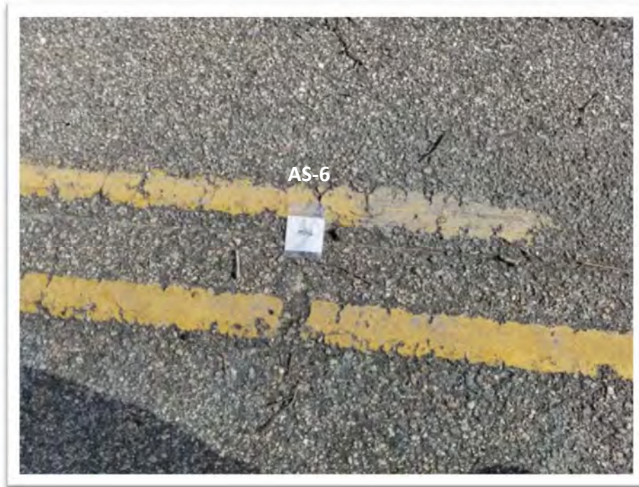
Photograph #21 Sample AS-6 – Asphalt Sampling Point on the Southwest End of Bridge 3 (None Detected)
