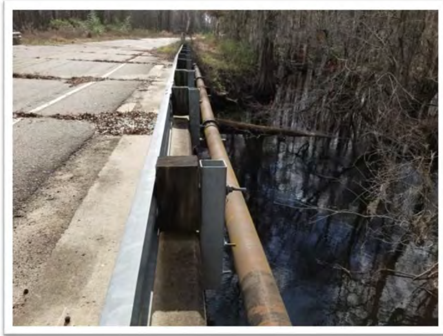
Photograph #13 View of Water Line Along the South Side of Bridge 2 – Looking Southwest
