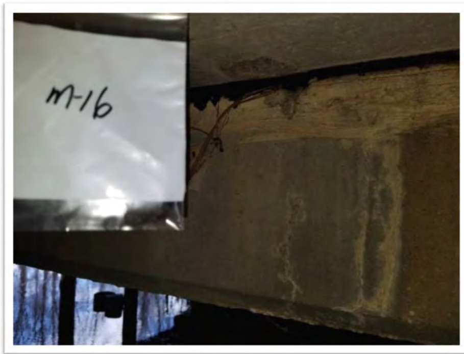
Photograph #24 Sample M-16 – Black Mastic Sampling Point Between Concrete Beams and the Black Bearing Pad on the Underside of the Deck on Bridge 2 (None Detected)
