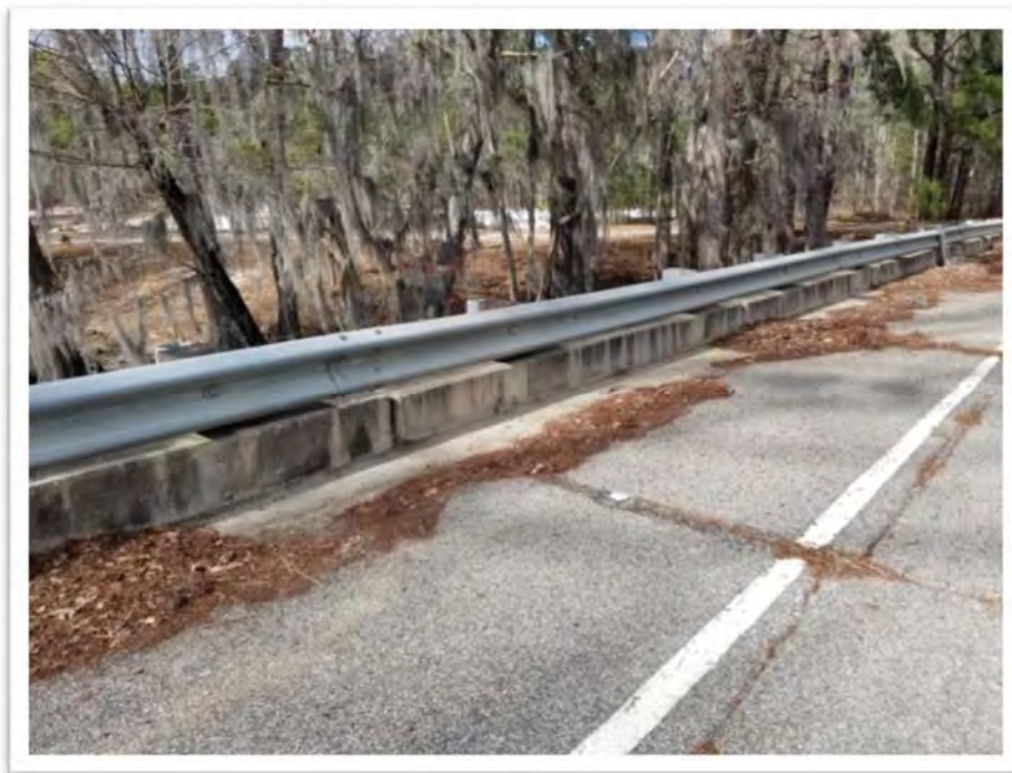
Photograph #19 View of the Metal and Concrete Railing on Bridge 3 – Looking North
