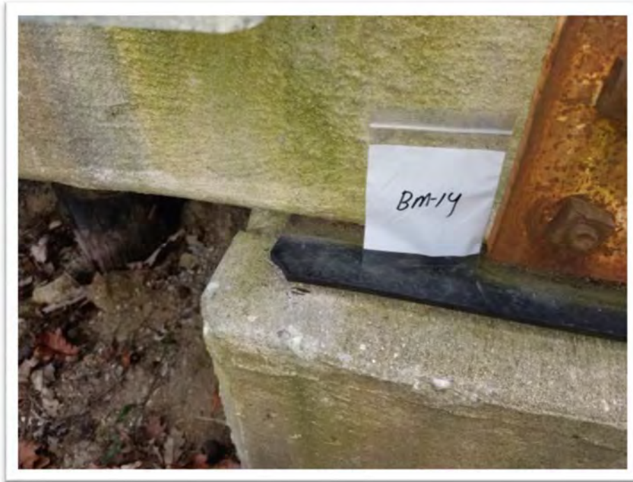
Photograph #23 Sample BM-14 – Black Bearing Pad Sampling Point Between the Deck of Bridge 2 and the Abutment at the Northeast End of the Bridge (None Detected)
